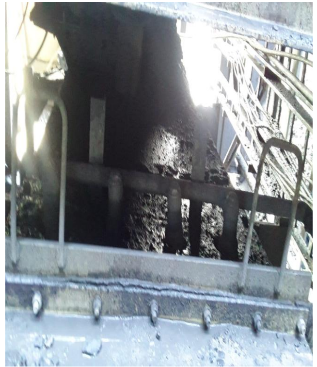
DSS sprinklers at BC-01 Tail end
