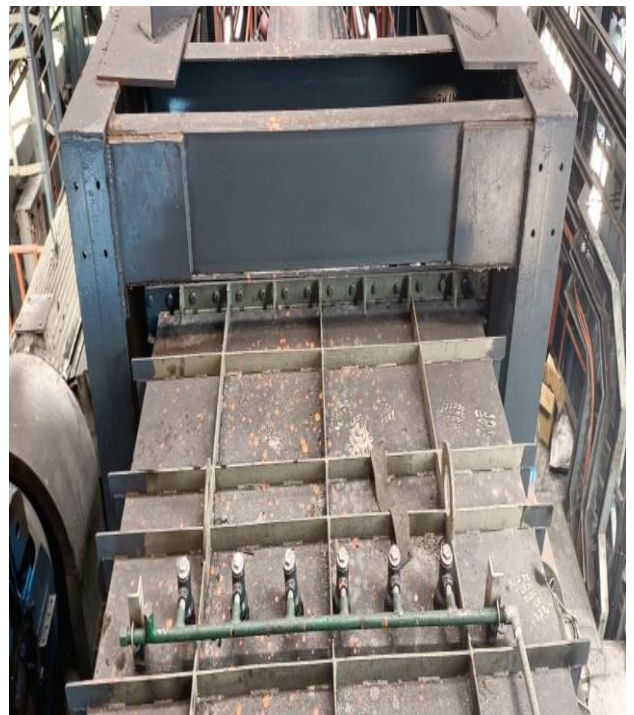
DSS sprinklers at PC Head end
