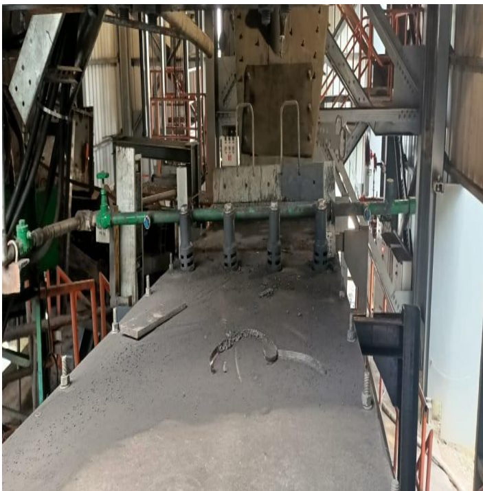
DSS sprinklers at BC-02 Tail end
