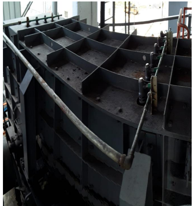
DSS sprinklers at Apron Feeder
